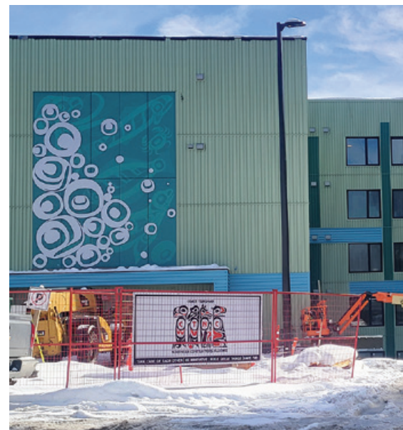
Figure 2 (below) 70-unit BC Housing Project led by Lax Kw'alaams WAAP Housing Society, Nearing completion in March 2026.
